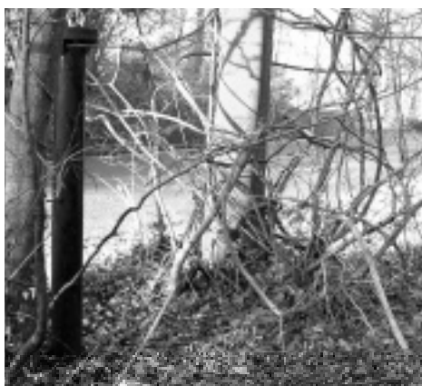
Breather pipe at crest of hill
